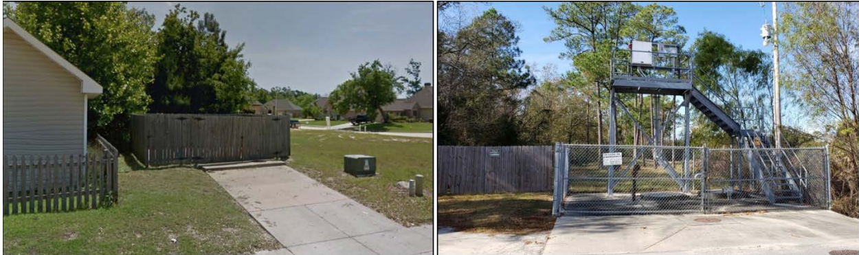
Figure 16. Lift station not located in a flood zone (left) compared to a lift station located in a flood zone that had to be elevated (right). Both are in residential areas.
