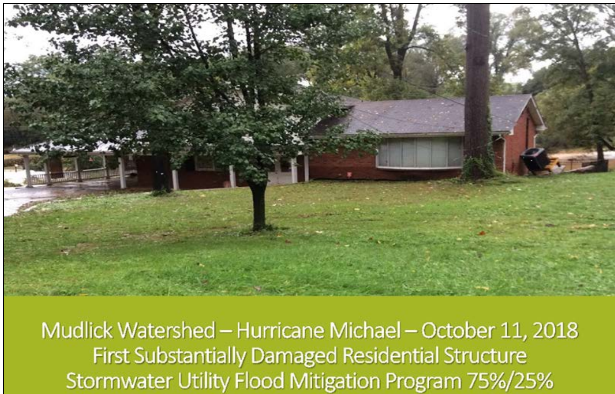
Figure 21. The first substantially flood-damaged home in Roanoke, which also prompted the city to implement an innovative approach to property acquisitions.
