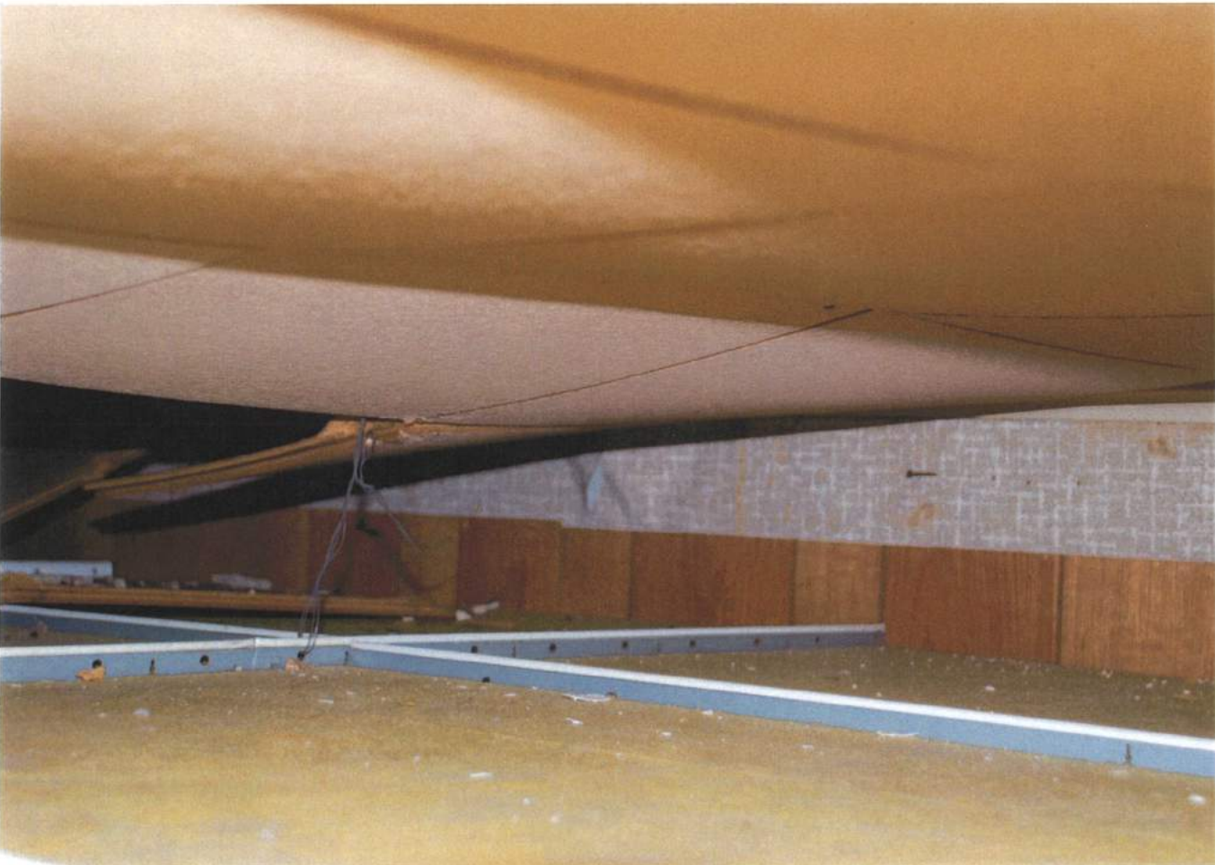
Space above suspended ceiling above second floor. Showing paneling, ceiling system, wallpaper and 20 th century Cellotex ceiling tile installation.
