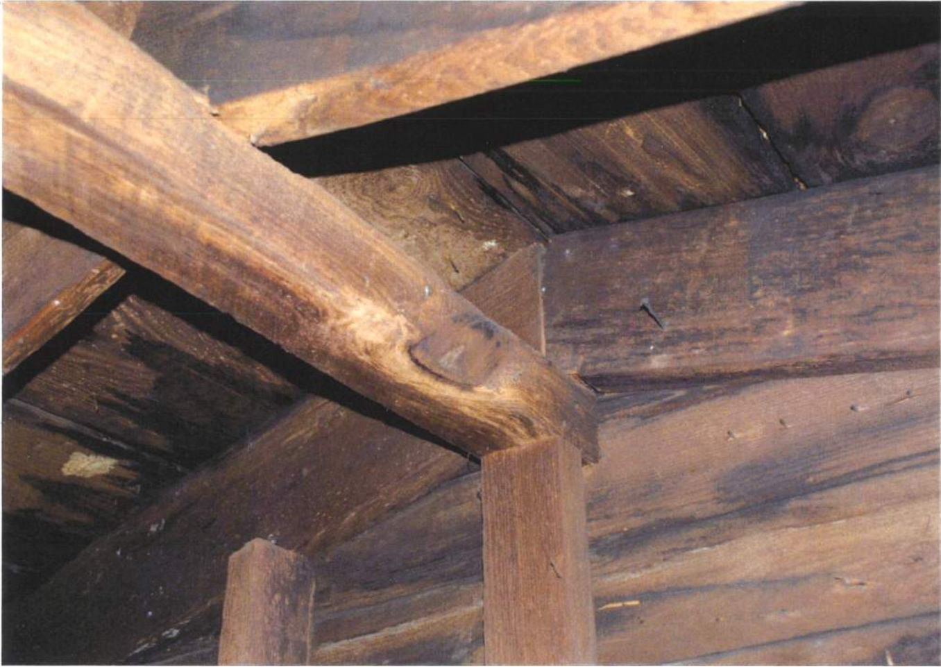
Attic framing showing ridge beam and rafters and inside surface of original exterior german siding. Looking northeast.
