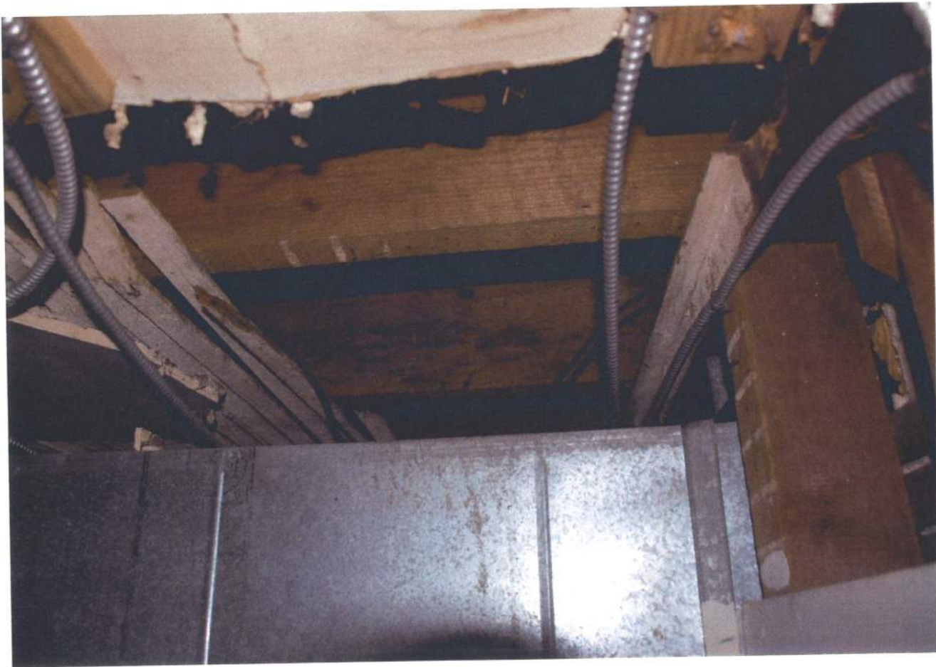
Space above suspended ceiling on First Floor. Showing ductwork, cables, and removed finishes.
