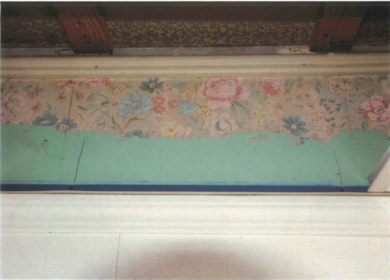
Space above suspended ceiling above large room on second floor. Showing early wallpaper and picture rail trim, papered ceiling, and furring for celotex ceiling tile.
