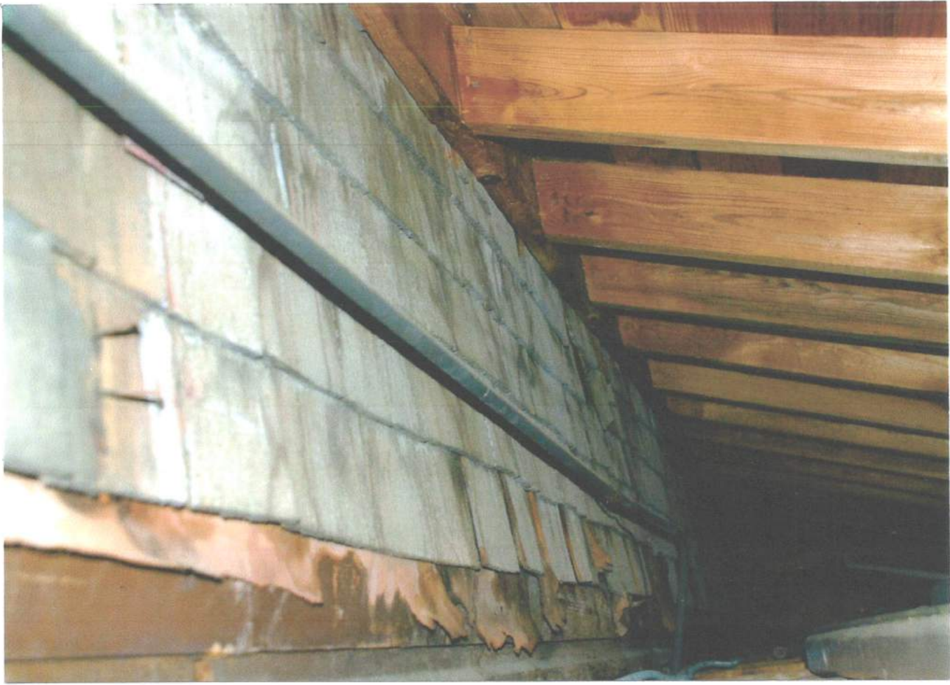
Roof structure above porch on southeast elevation. Showing 20 th century porch framing set on shingle siding (installed over original German siding.)
