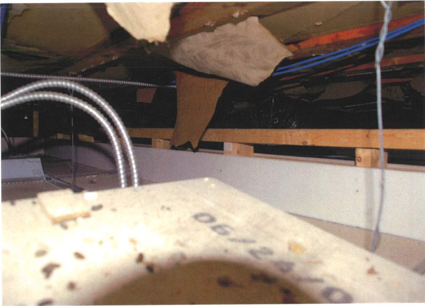
Space above suspended ceiling on First Floor. Showing new framing and drywall.
