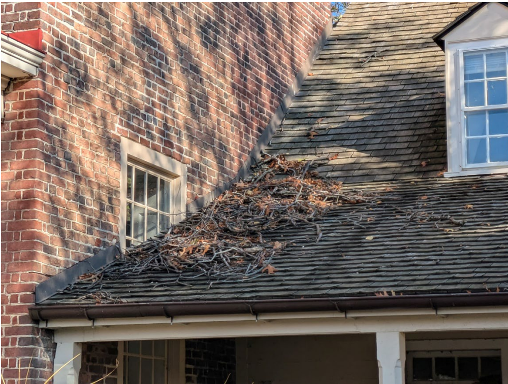
Adjoining roof between mid-18th-century log house and early-19th-century Federal-style brick wing, showing displaced materials from egret's nest on brick wing chimney.
