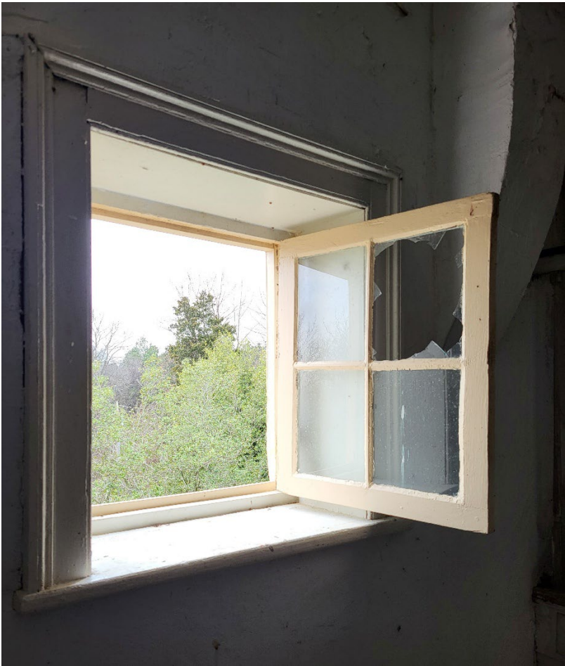
Damaged attic window.
