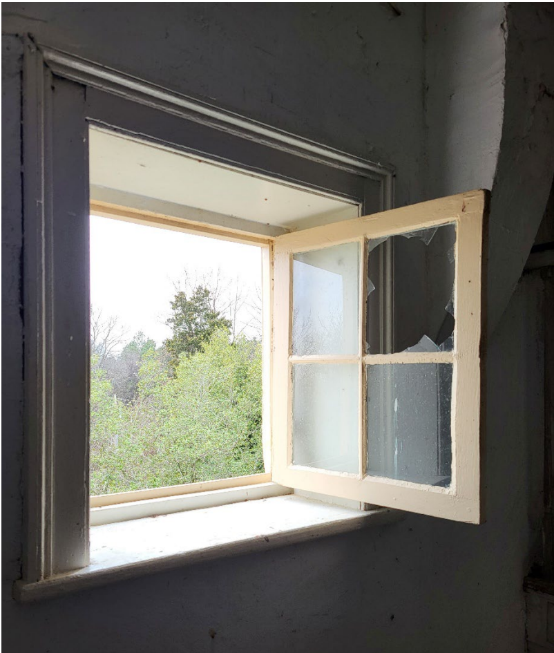
Damaged attic window.
