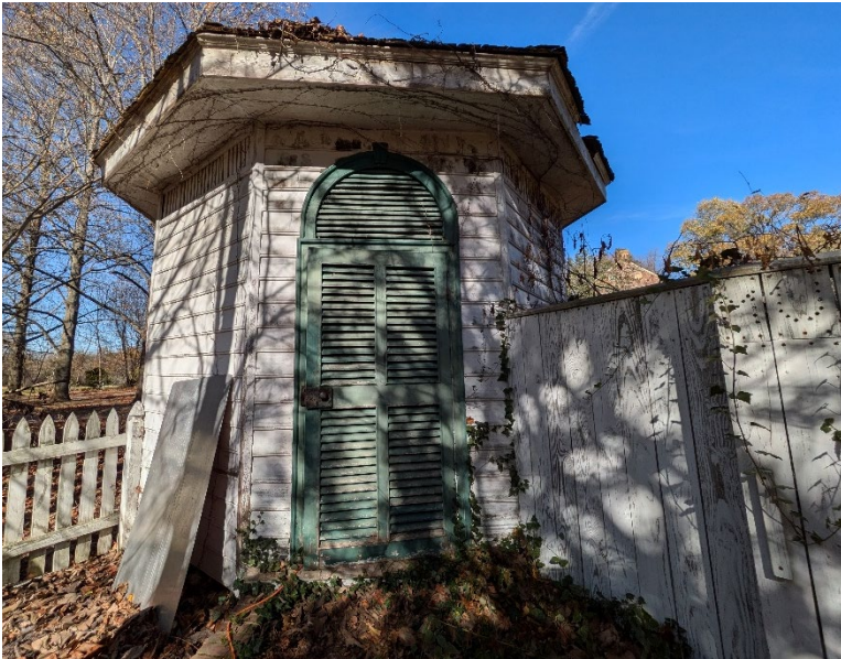
Dairy, requiring repair.
